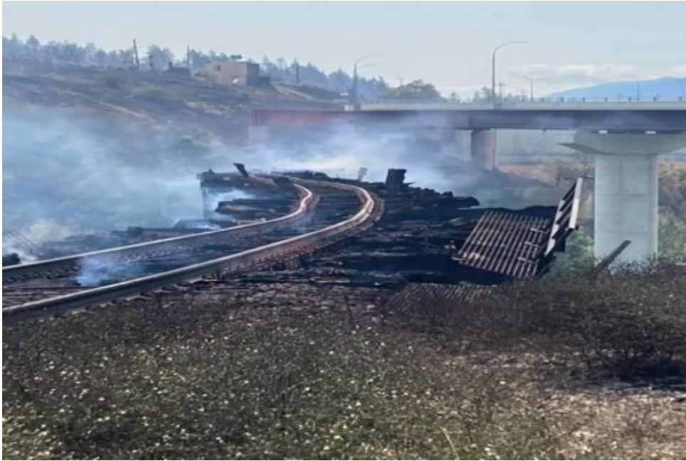
Burnt out CN Lytton Bridge
